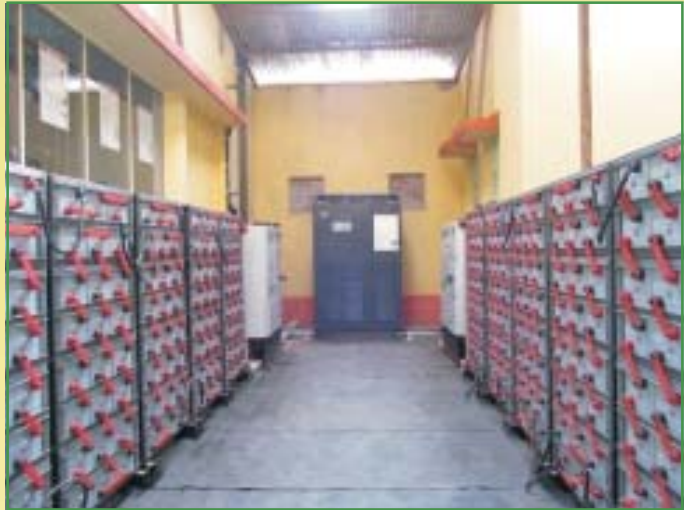
Solar Inverter and Battery Back-up
