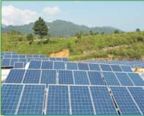
Solar Panels of NIT-Arunachal Pradesh [This is reportedly the first of its kind among the thirty (30) NITs]
