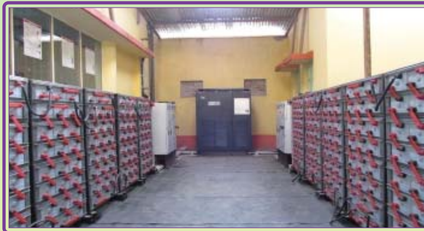
Solar Inverter and Battery back-up
