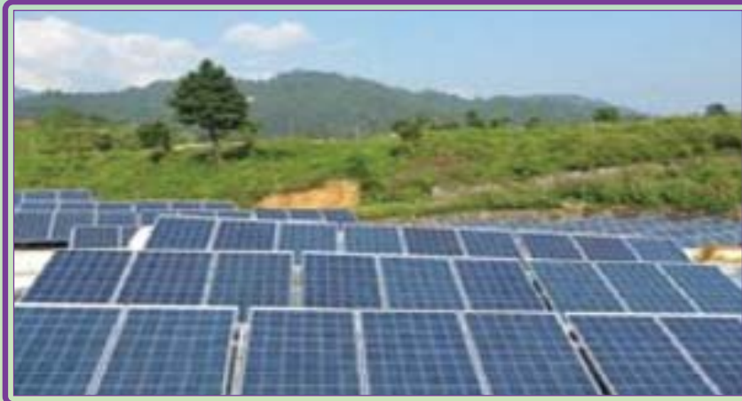
Solar panels of NIT- Arunachal Pradesh [This is reportedly the first of its kind among the thirty (30) NITs]
