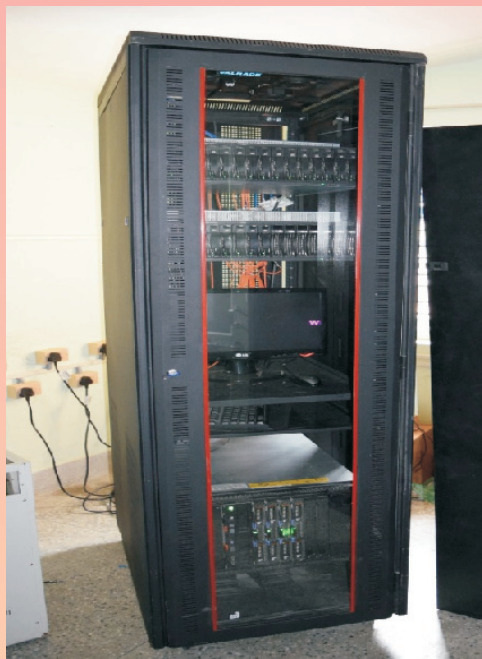
IBM Blade servers & IBM Storage
