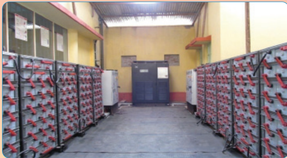
Solar Inverter and Battery back-up
