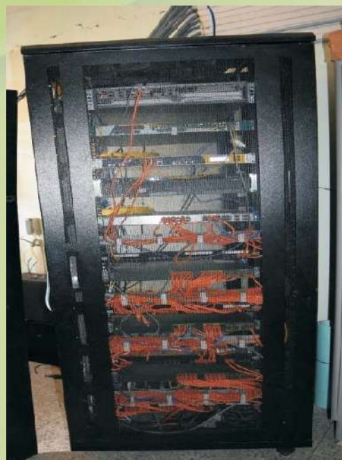
Firewall, Router Layered (L3&amp;L2) Switches
