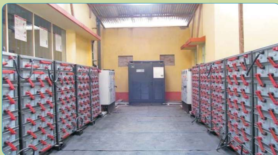
Solar Power Control Room
